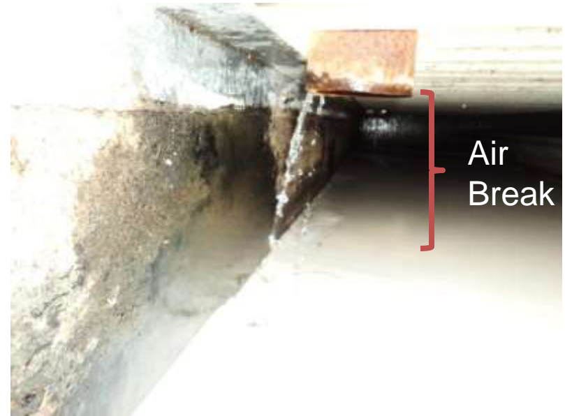
City make up enter Tomkins Tower via air break configuration
