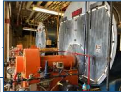
Boilers 22 yrs old
