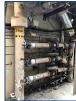
Steam Piping Needs renewal within 10 yrs
