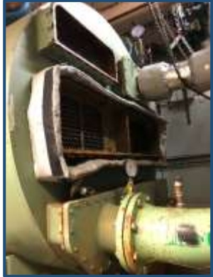
Abs. Chiller Over 30 yrs old
