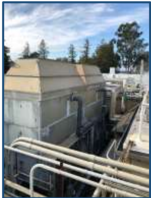
Cooling Tower Poor condition
