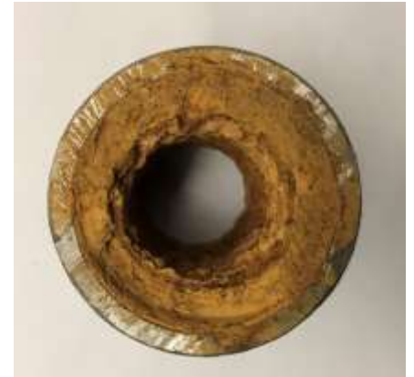
Figure 10: Residue in the Pipe (UI Energy plant)
