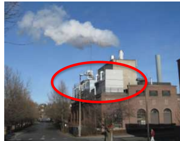
Figure 2: The cooling towers (on the roof) for the district heating and cooling plant
