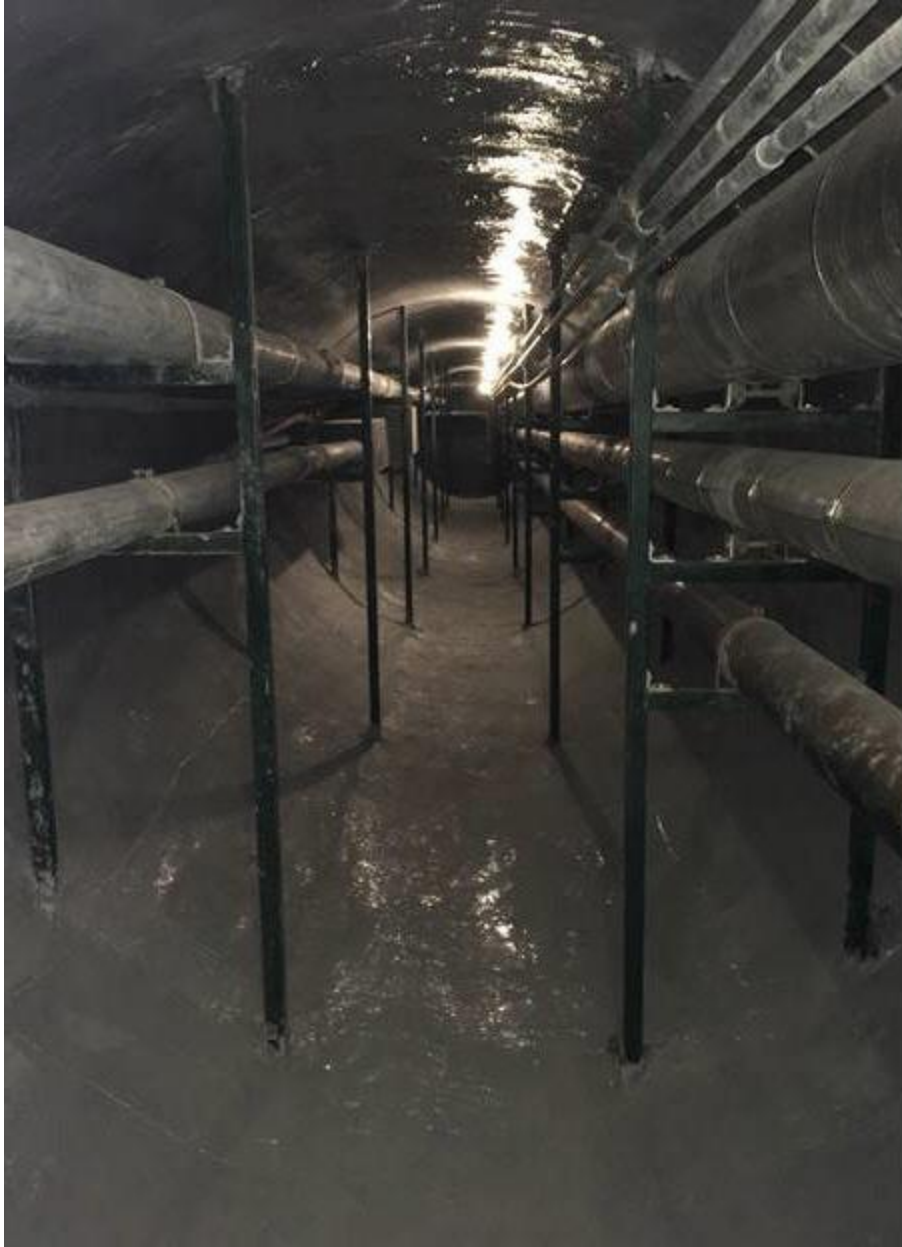
Caption 2: After: Inside repaired utility tunnel under the University of Arizona campus.
