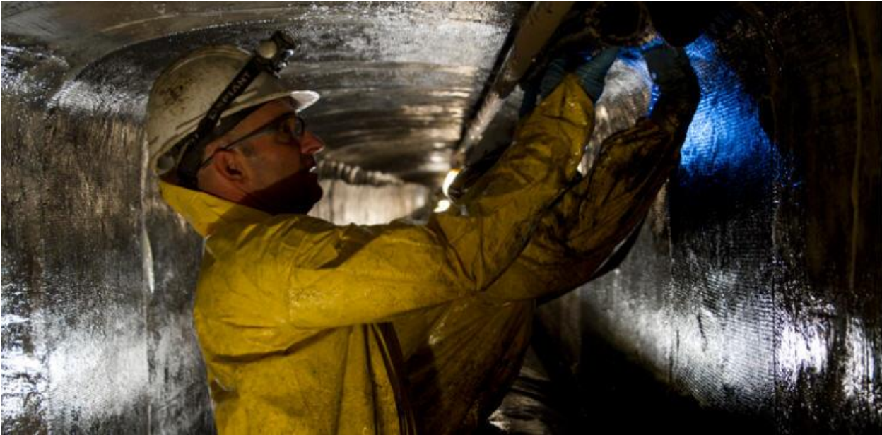
Figure 1: Before: Workers apply carbon fiber mats soaked in epoxy resin to stabilize the tunnels that crisscross under the University of Arizona campus.
