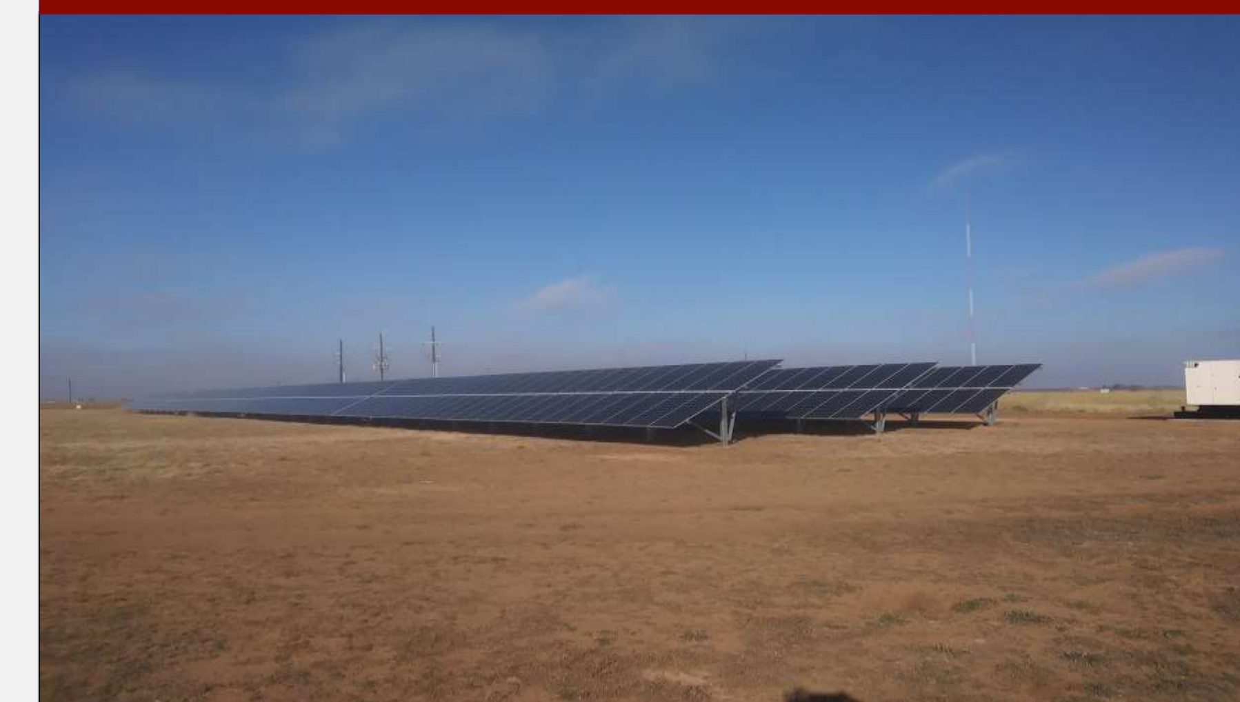
Figure 5: 150 kW solar array
