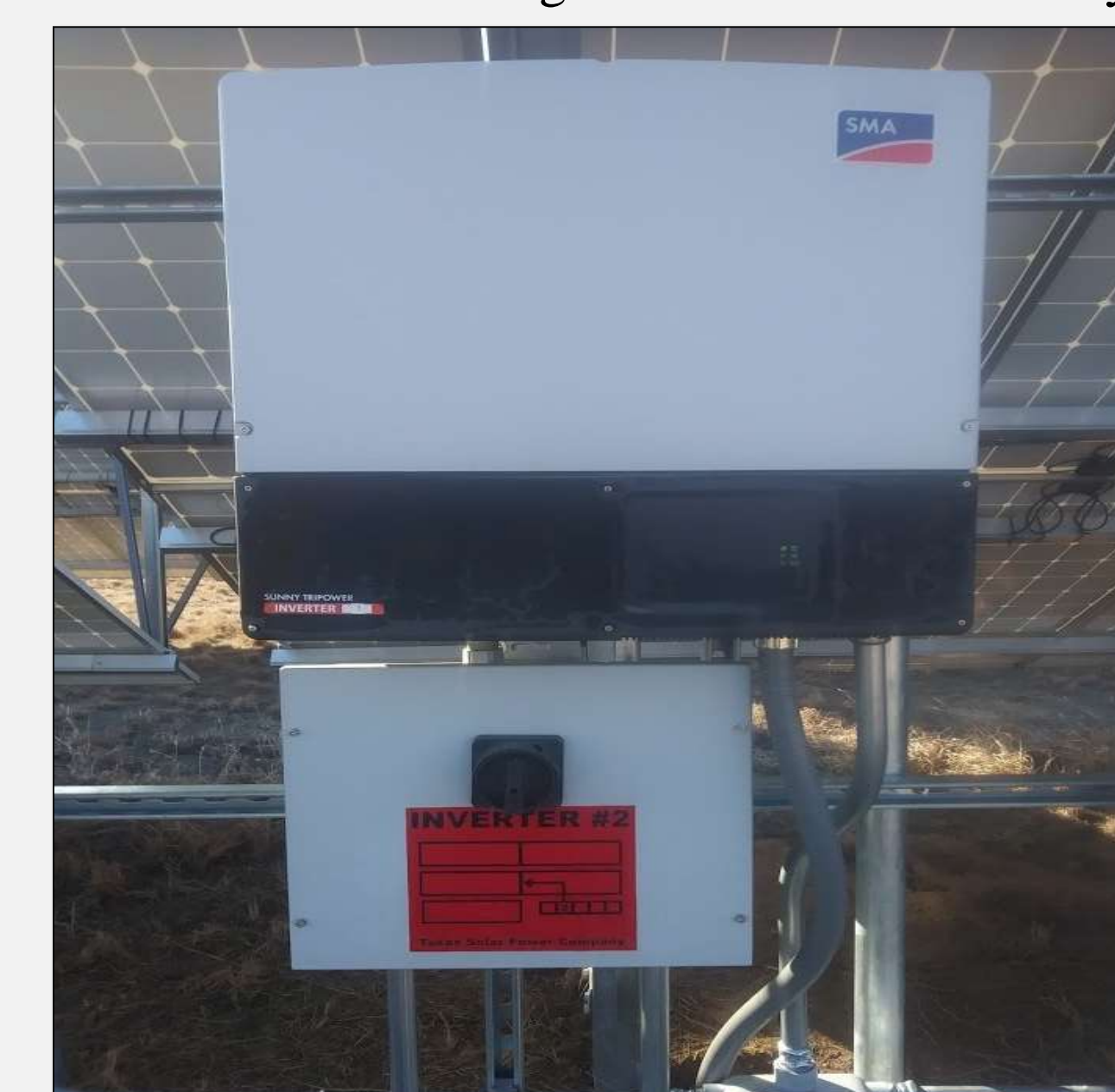
Figure 8: 30 kW solar inverter
