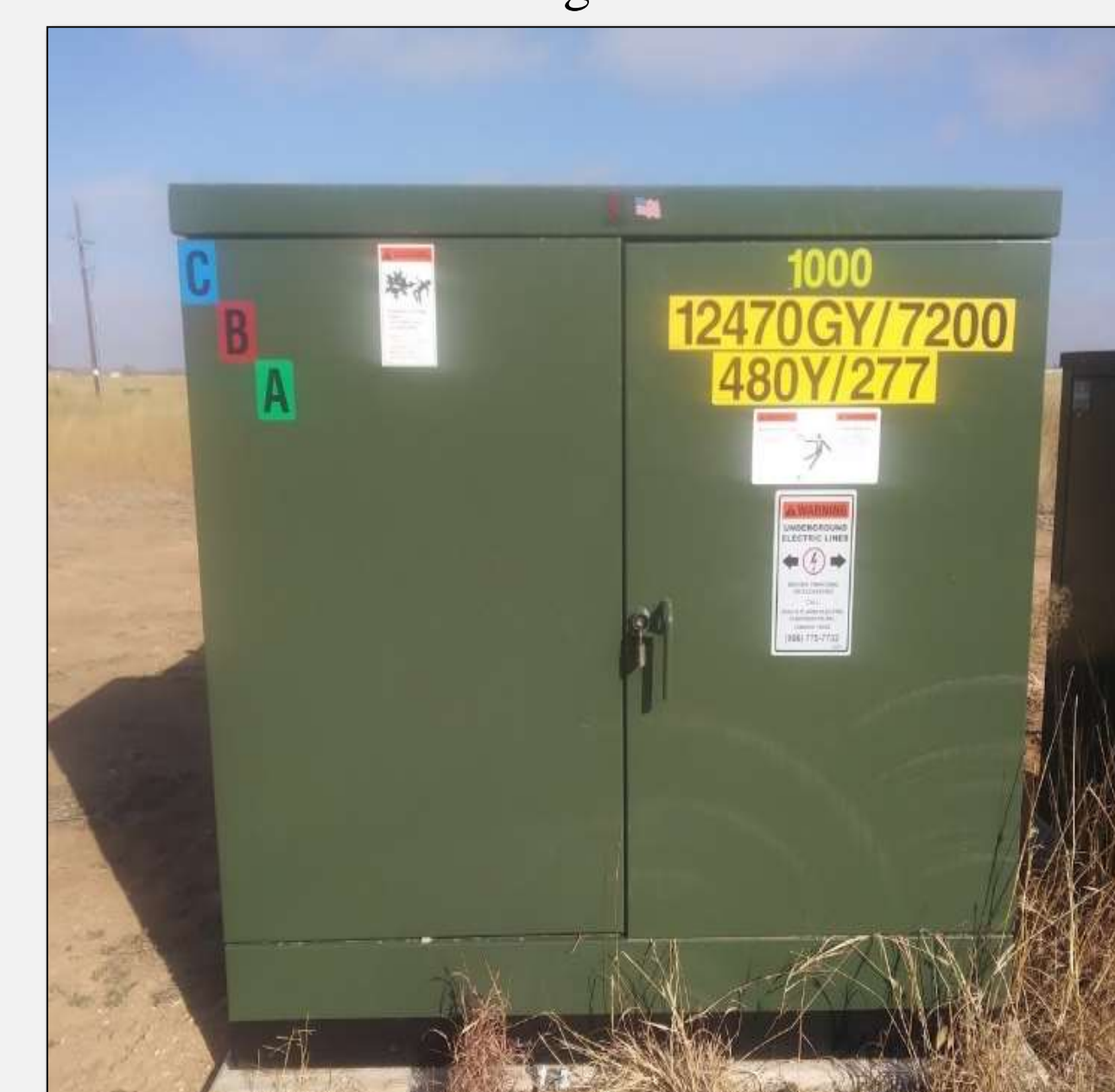
Figure 9: Step up transformer
