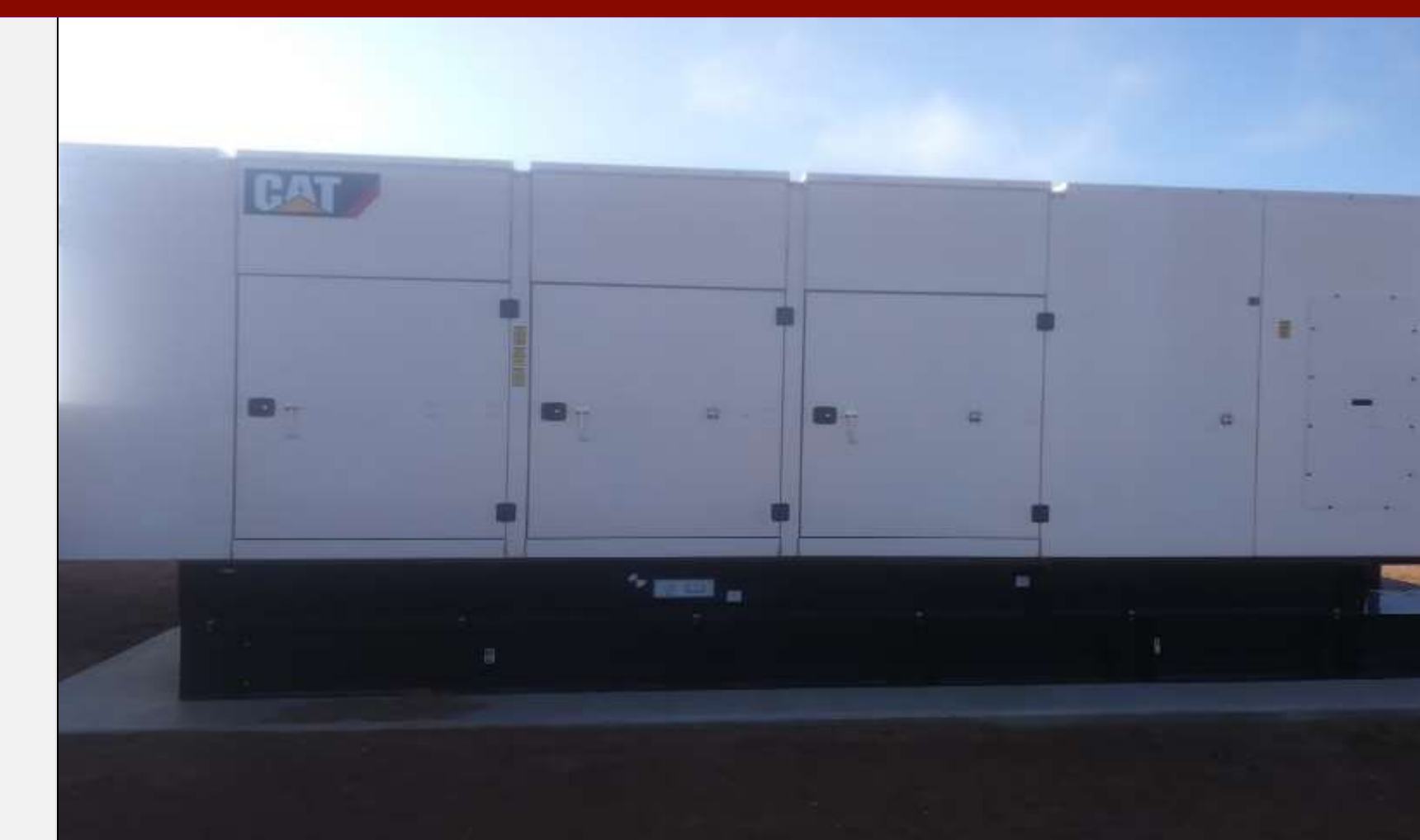
Figure 7: Tier 4 diesel generator
